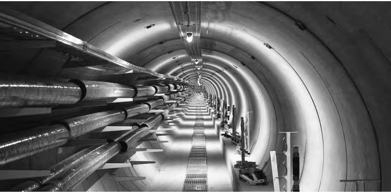
Image: Tunnel with cables under the railway station, beuret.net, 2024.
