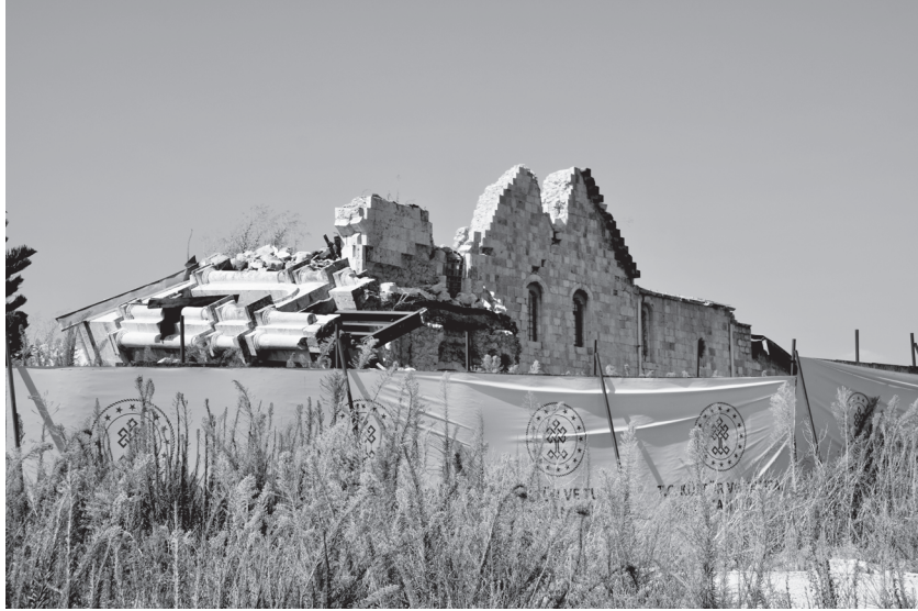
Fig. 26: St. Paul's Church after the earthquake, August 29, 2024.
