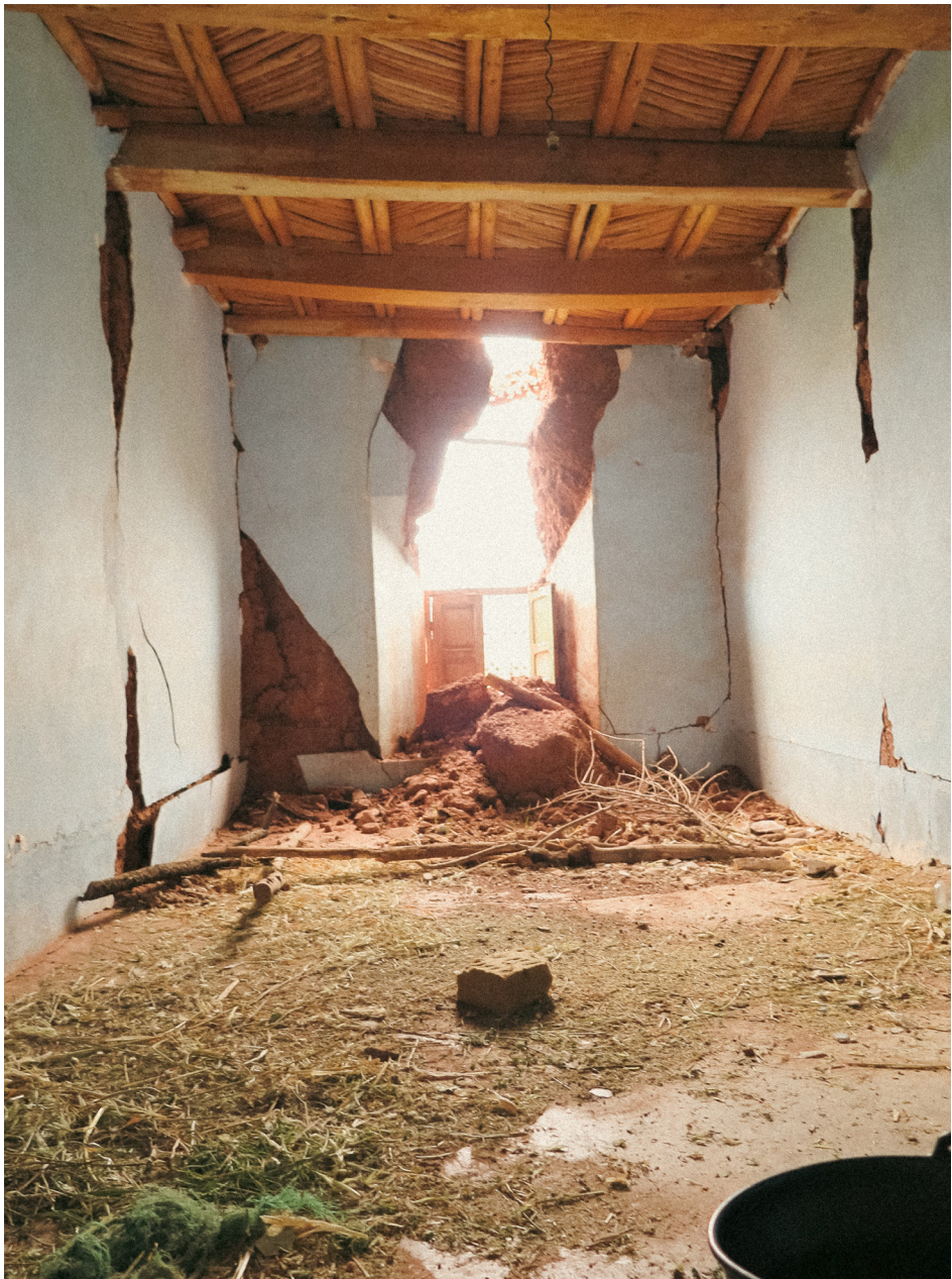
Collapse at window opening and beam supports, common structural weak points Ouirgane, October 14, 2024
